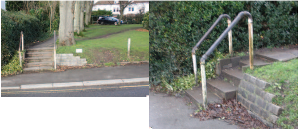
Fig 2.3 – Worn Grass Area and Poor Standard Steps
