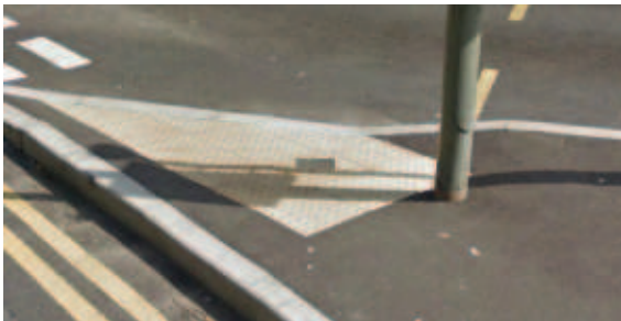
Fig 10.1 – Lighting Column Obstructing Pedestrian Movements on Wellhouse Lane
